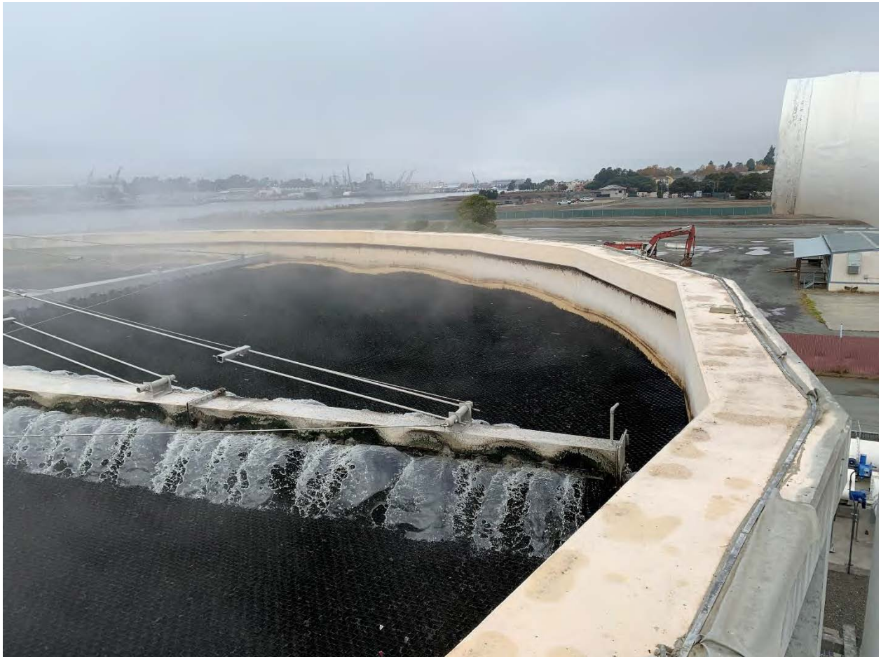
Vallejo Flood and Wastewater District treatment plant, highlighting one of two biotowers.
