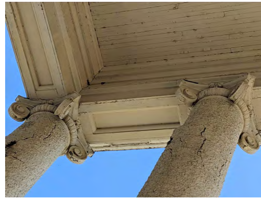
DAMAGED PORTE COCHERE DECORATIVE PLASTER COLUMNS AND WOOD PANEL BEAM SURROUND, SEE SHEET NOTES FOR SCOPE OF WORK INFORMATION
