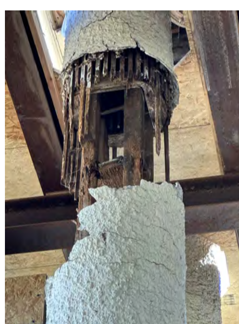
INDIVIDUAL DAMAGED PORTE COCHERE DECORATIVE PLASTER COLUMNS, SEE SHEET NOTES FOR SCOPE OF WORK INFORMATION
