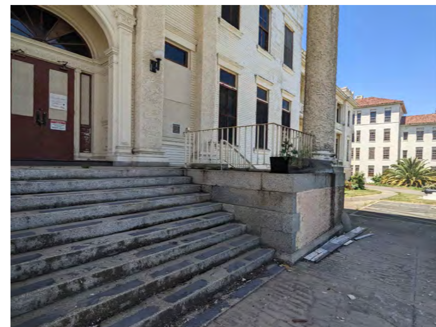
EXISTING EXTERIOR STAINED GRAND CONCRETE STAIR AND RUSTED DECORATIVE IRON GUARD RAILS, SEE SHEET NOTES FOR SCOPE OF WORK INFORMATION
