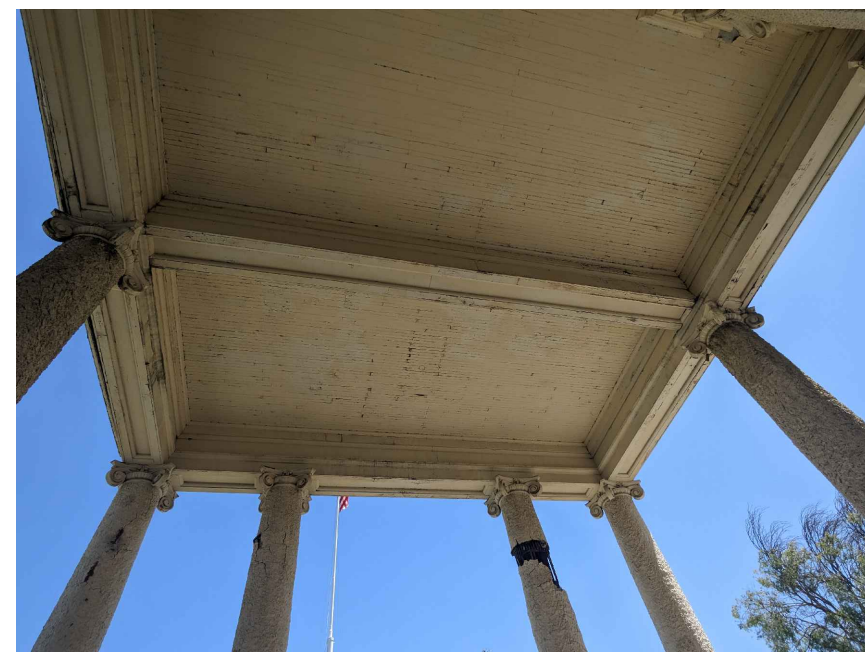
DAMAGED PORTE COCHERE DECORATIVE PLASTER COLUMNS AND CEILING STRUCTURE, SEE SHEET NOTES FOR SCOPE OF WORK INFORMATION
