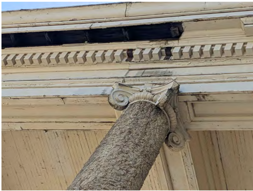
DAMAGE AND MISSING ORNAMENTAL WOOD CORNICE, DENTILS, FRIEZE, ARCHITRAVE, COLUMN CAPITALS AND WOOD PANEL BEAM SURROUND, SEE SHEET NOTES FOR SCOPE OF WORK INFORMATION
