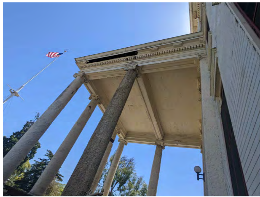
DAMAGED ORNAMENTAL WOOD CORNICE, DENTILS, FRIEZE, ARCHITRAVE, SEE SHEET NOTES FOR SCOPE OF WORK INFORMATION
